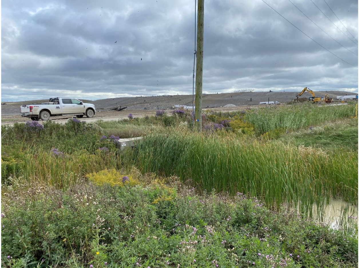
Image looking east shows the inlet structure of the SWM pond with Street 'C' in distance.
