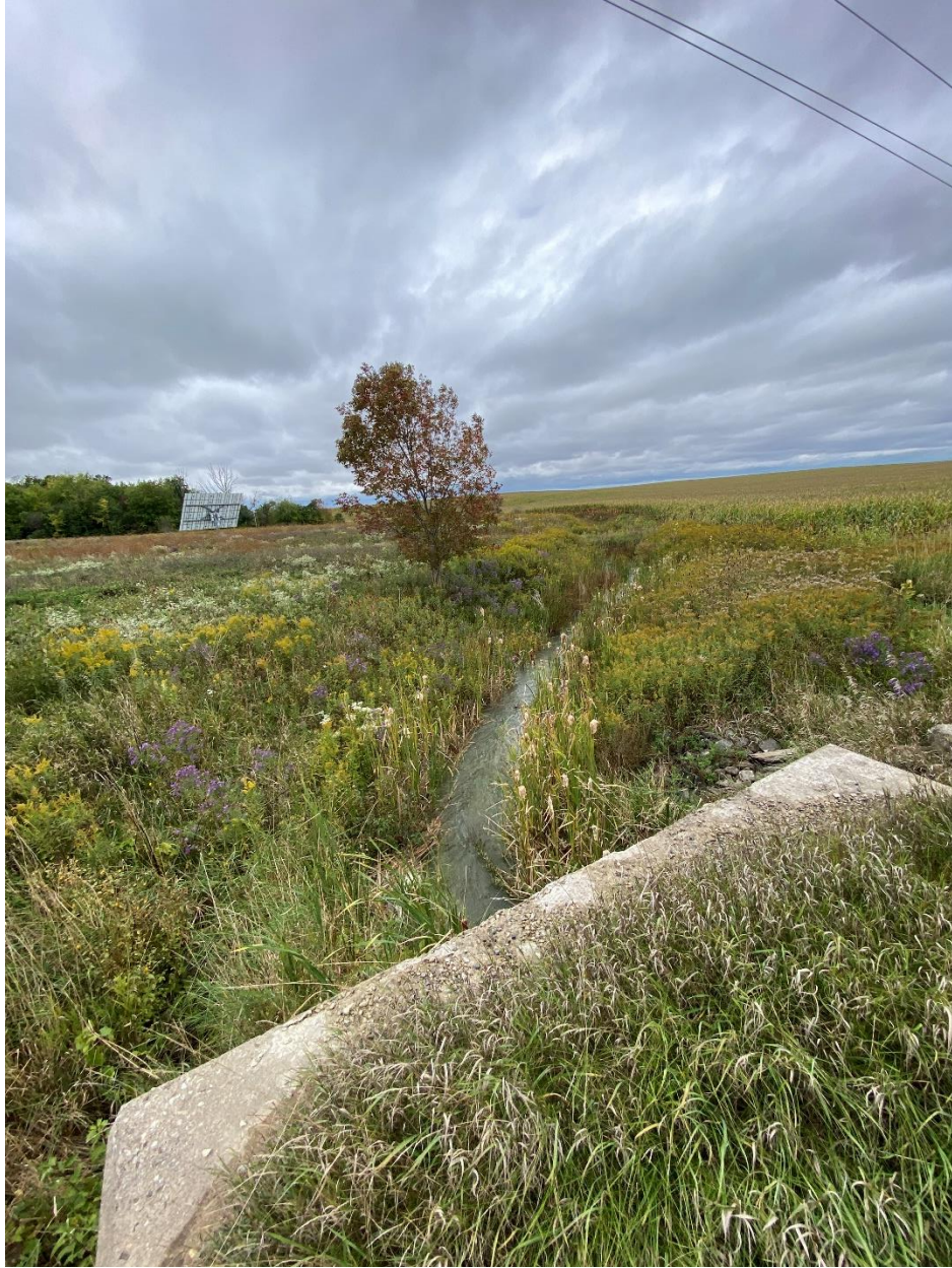
Nauvoo Road culvert looking west (downstream) outlets into the Gilliland Geerts Drain.
