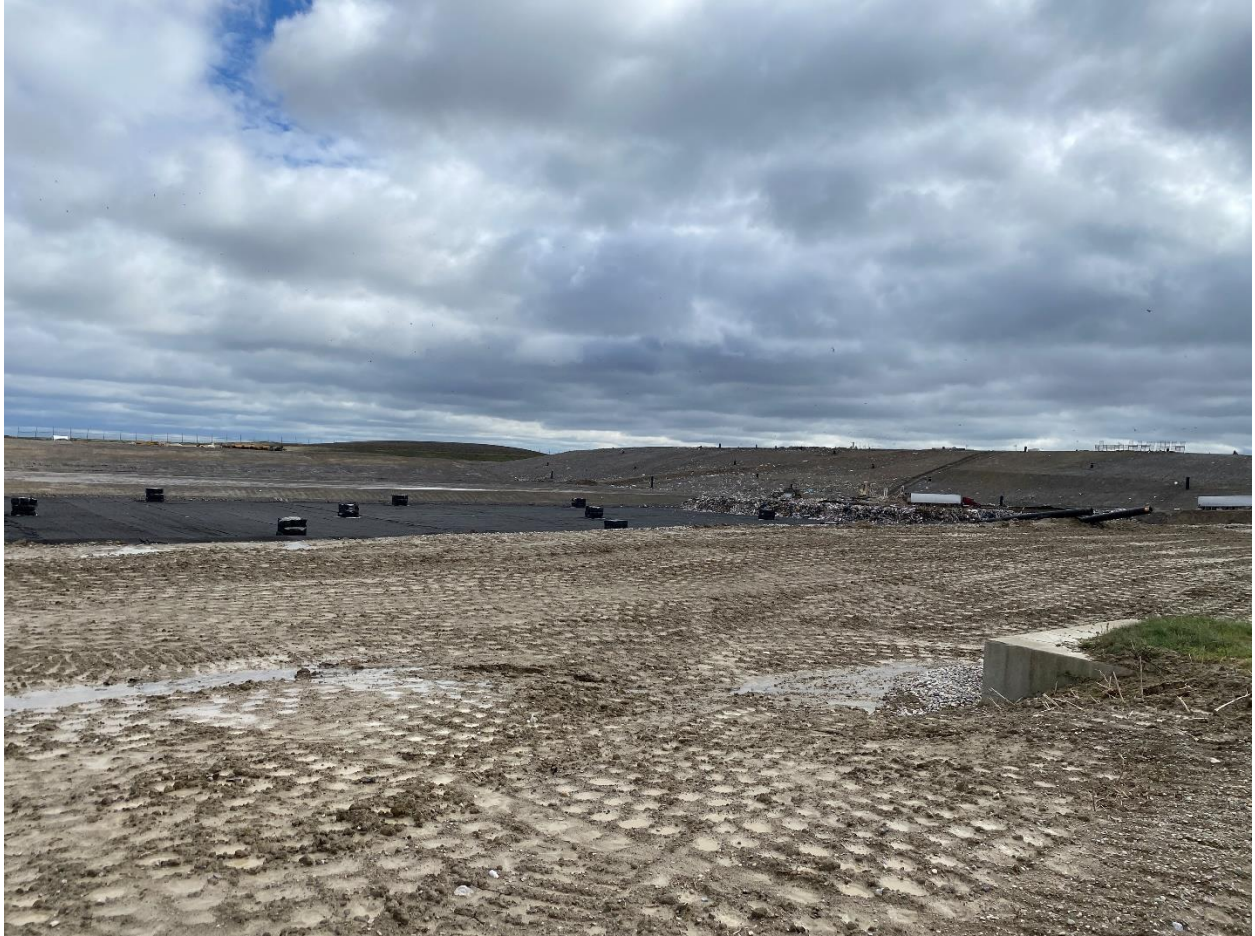
Image looking west shows the expansion area of the site and the reinforced concrete box culvert that acts as an inlet structure for the SWM Pond 3.
