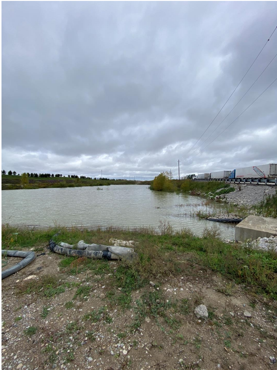
SWM Pond 2 located in the southwest corner of the site. Image looking northwest shows inflows into the pond from the reinforced concrete box culvert near Street 'C'.
