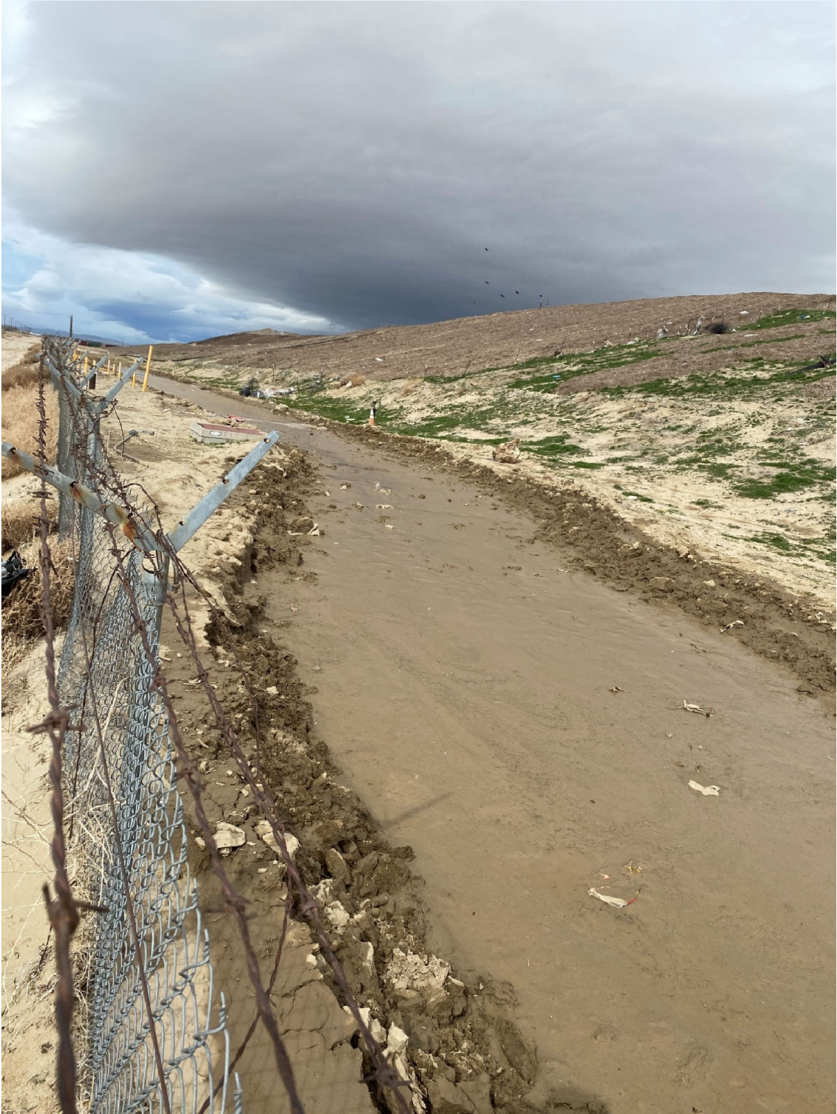
Photo 5: Ponding water southern perimeter looking west.
